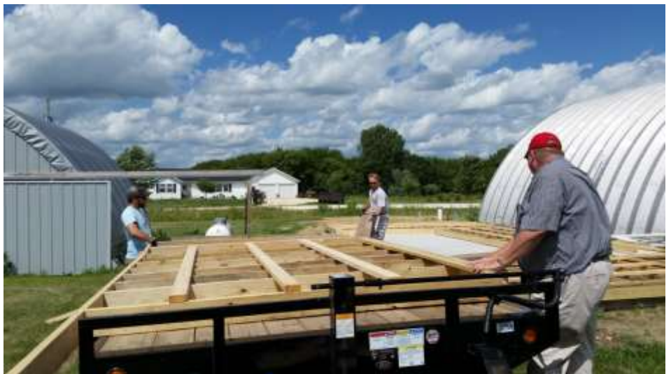
Left – Fred Lansing works on sewer. Rt.- Ron Radloff delivers wall he built
